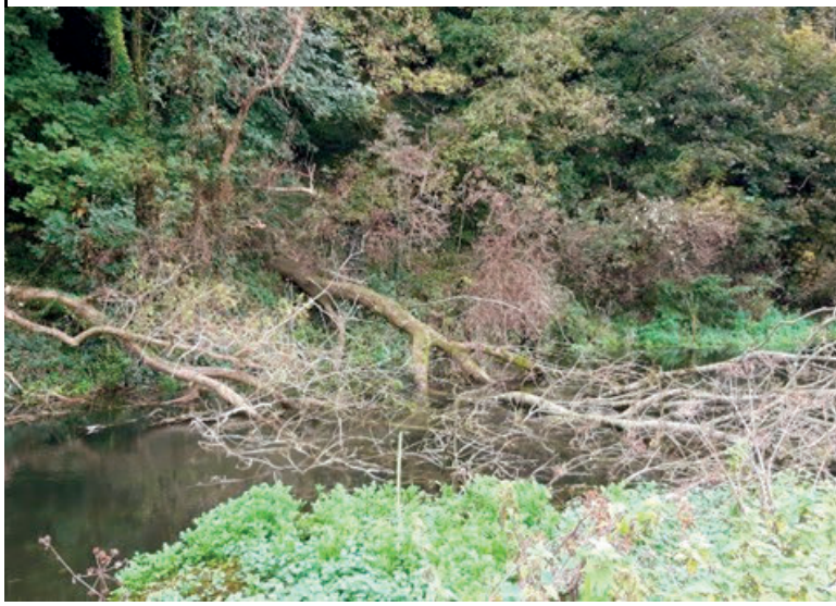
Trees were felled along a steep bank to allow more light into the over shaded river channel. Trees of low ecological value were chosen.
